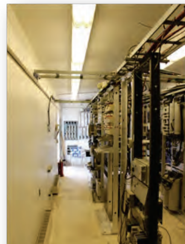
Figure 3-3. Example Equipment Racks - Caltrans Shelter
