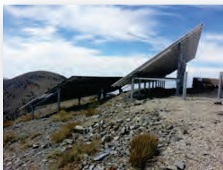
Figure 3-1. SCE and USAF Solar Arrays
