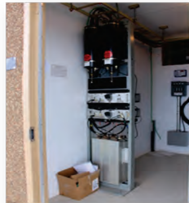
Figure 3-7. Example Equipment Racks NPS Shelter
